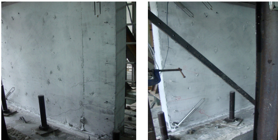
Figure 3.19. Initial Diagonal Cracks (T5-S1).
