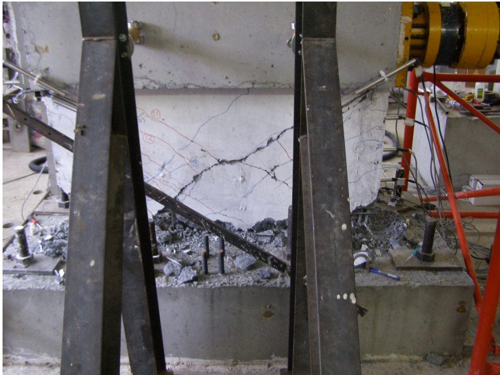
Figure 3.26. High Damage Level (T1-S2).
