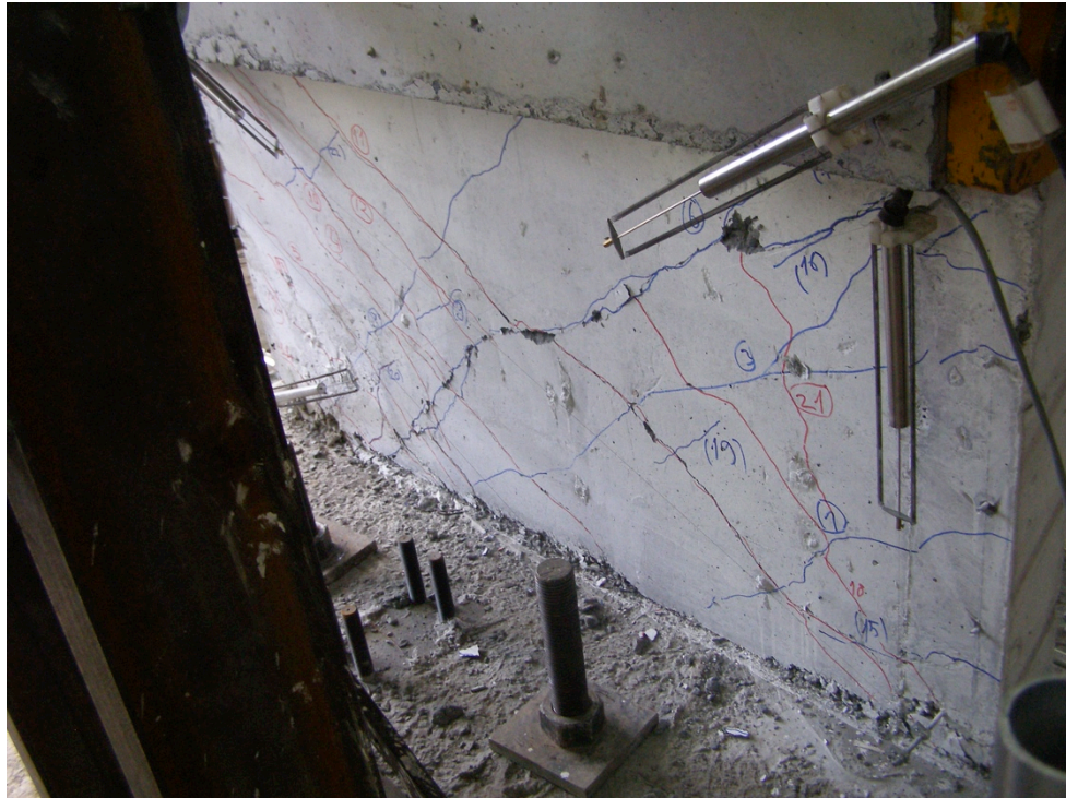
Figure 3.25. Main Diagonal Crack at Ultimate Load (T1-S2).
