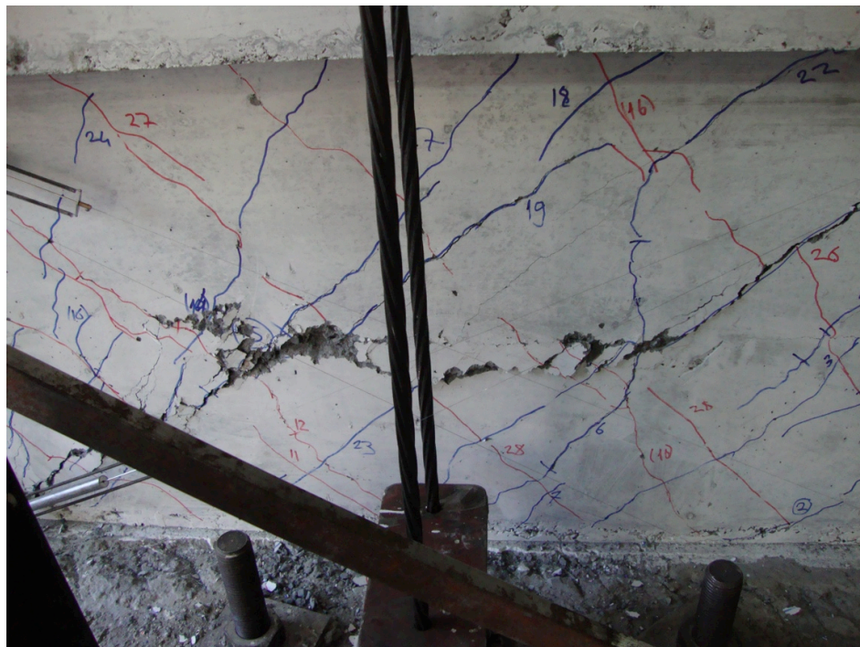
Figure 3.28. Main Crack (T1-N10-S1).
