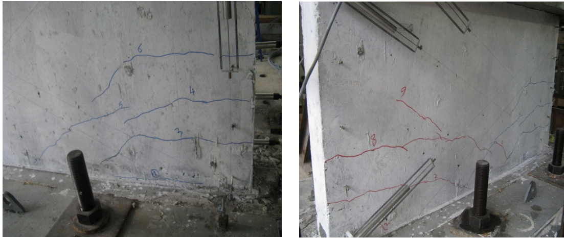
Figure 3.13. Initial Diagonal Cracks (T3-S1).
