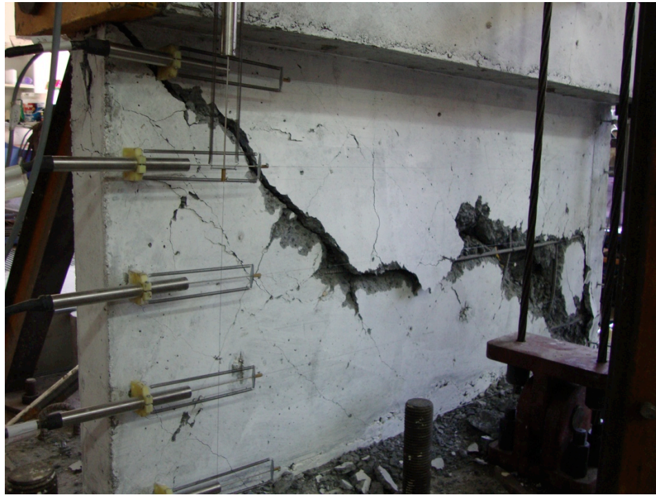
Figure 3.29. High Damage Level (T1-N10-S1).
