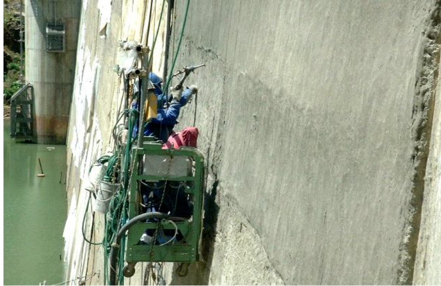
Figure 2.15 Spray repair of the Mitaka Dam with ECC for water-proofing (Sakata et al., 2004)
