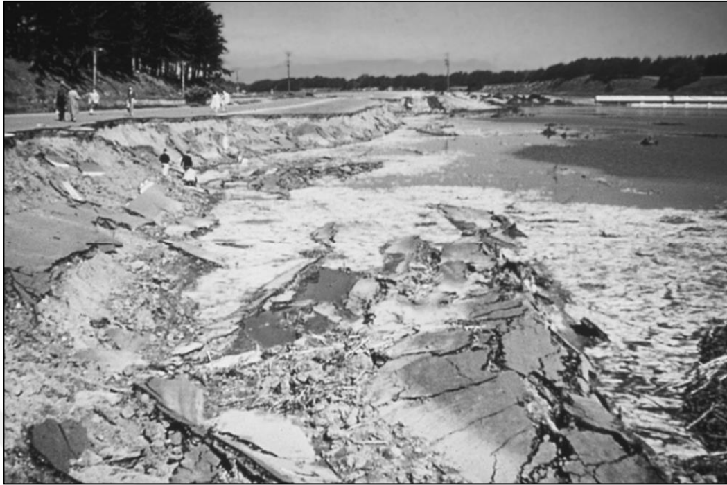
Figure 2.2 A small flow slide along the shore of Lake Merced in San Francisco in 1957.(Kramaer,1996)
