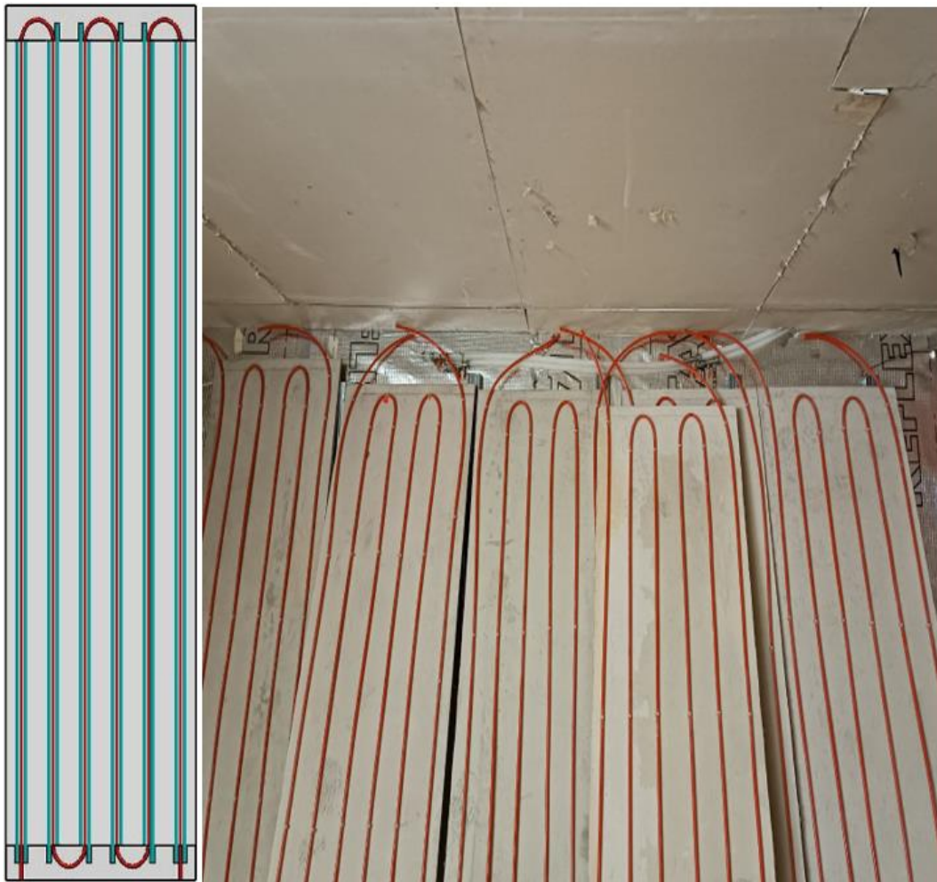
Figure 3.34 New panel view
