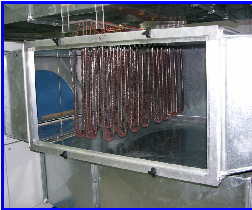
Figure 3.10. The photographic view of electric heater unit
