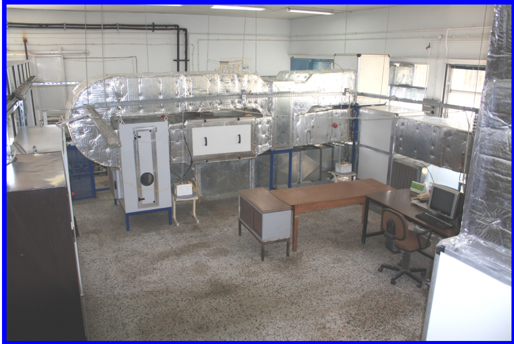
Figure 3.11. The photographic view of desiccant cooling system
