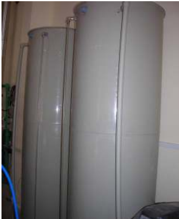
Figure 2.1 Geothermal water storage tanks
