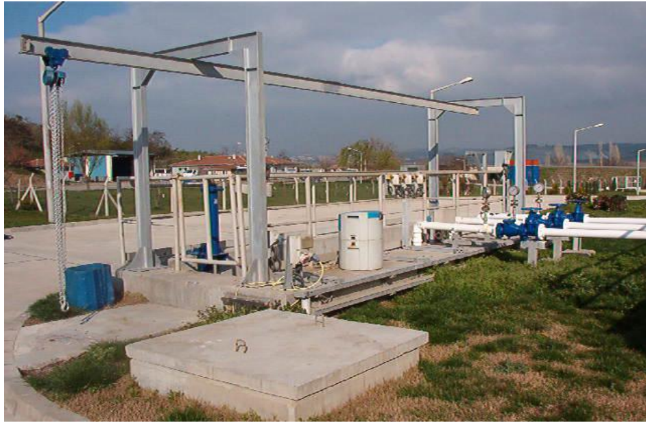
Figure III. 4 The pumping station
