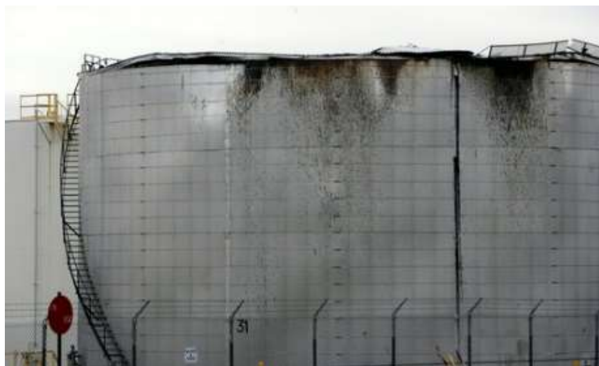
Figure 2.4 Roof damage of storage tank
