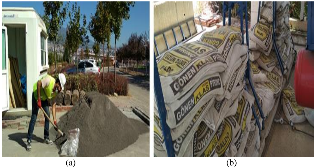
Figure 3.8. (a) Filling slag in the bag, (b) Placement of slag into bag inside barrier.
