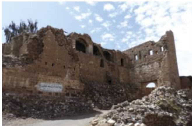
Figure 4.3. Kawkaban city gates, destroyed by aerial bombardment carried out by the Saudi-led coalition,Source: Sarah Rijziger, 2017.
