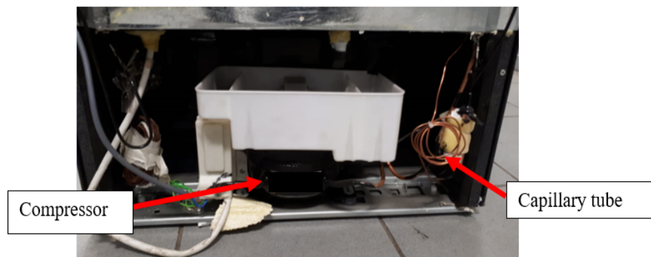
Figure 6.4. Machine room of the refrigerator.
