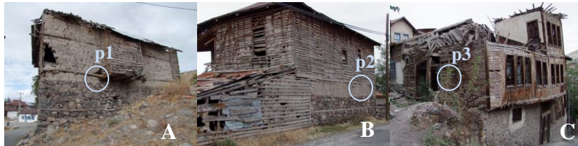
Figure 3.36 The locations where the material samples were taken from the traditional timber frame houses (A) and (B): in the village of Kavaközü with the door numbers 15 and 39 respectively; (C) in Beypazarı.
