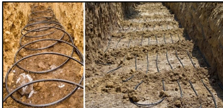
Figure 2.5: Geothermal Energy installation (Krietsch, B, 2020)
