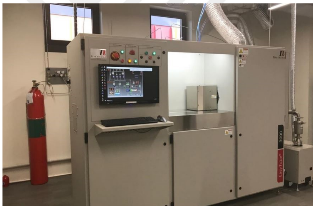
Figure 2.2: A model CVD reactor room for advanced manufacturing.
