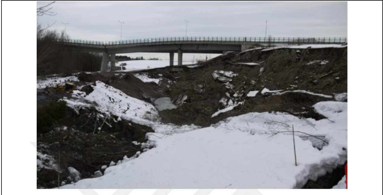
Figure 2.1: Bridge Damaged by Landslide, Norway [19]
