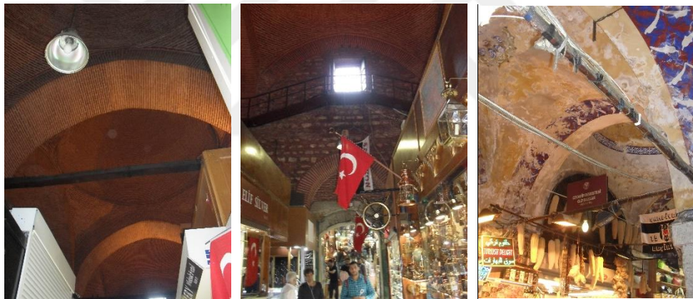
Figure 4.28 (a) Lightening tools inside the bedesten, (b) Cevahir Bedesten's windows, (c) electricity cables in the bedesten's one leading street, taken by author on 18.10.2016
