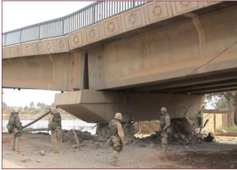
Figure 3. A Bridge in Iraq Damaged by an Explosion [2]
