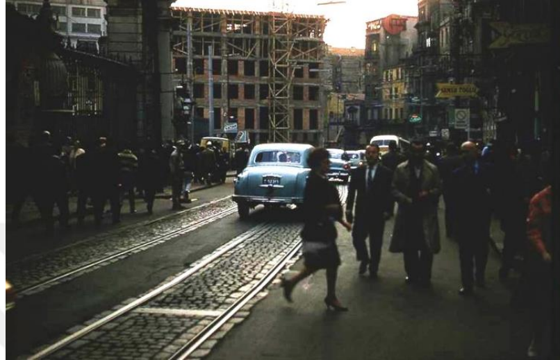
Figure 2.8. Construction of the Yapı Kredi Bank Building, early 1960s, Teget Architects' Archive
