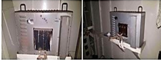
Picture No 1. Dry Type transformers in Engine Room.
