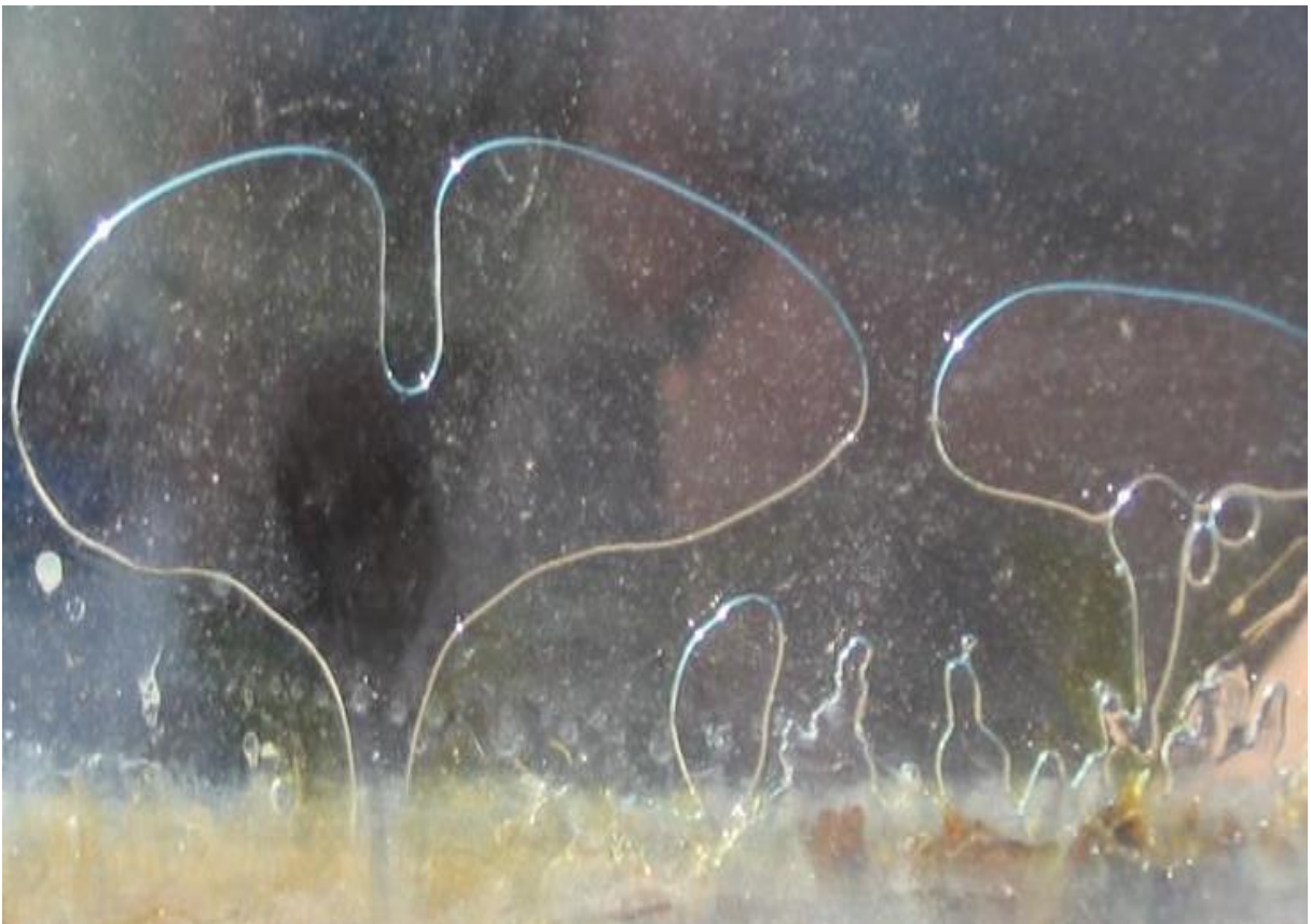
Picture 1.3 Delaminated glass window
