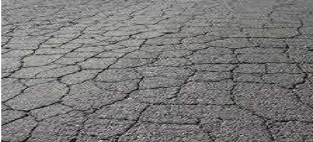
Figure 2.1. Fatigue cracking (Aziz, 2016)
