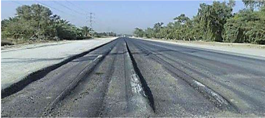
Figure 2.2. Rutting occurring in a road pavement in Iraq
