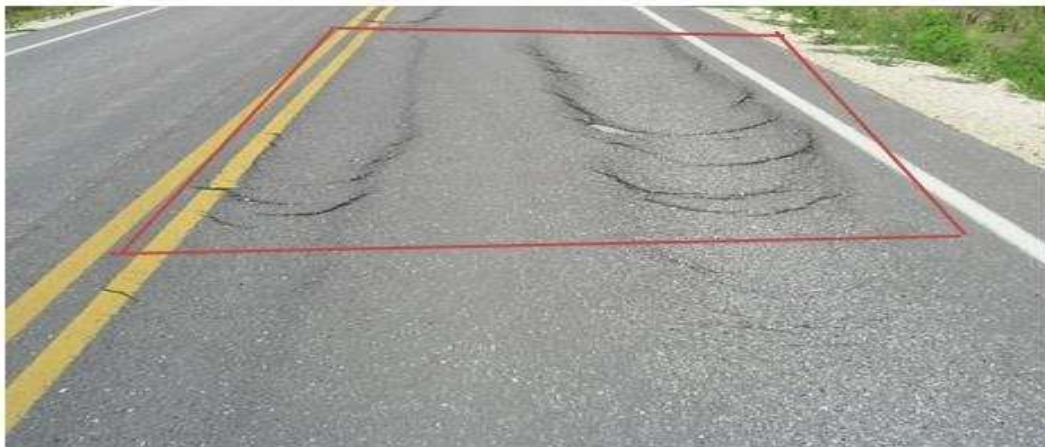
Figure 2.3. Shoving of an asphalt road pavement (Nuushuun, 2021)
