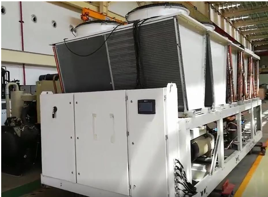
Fig. 2-1 The chiller used for experimental data collection
