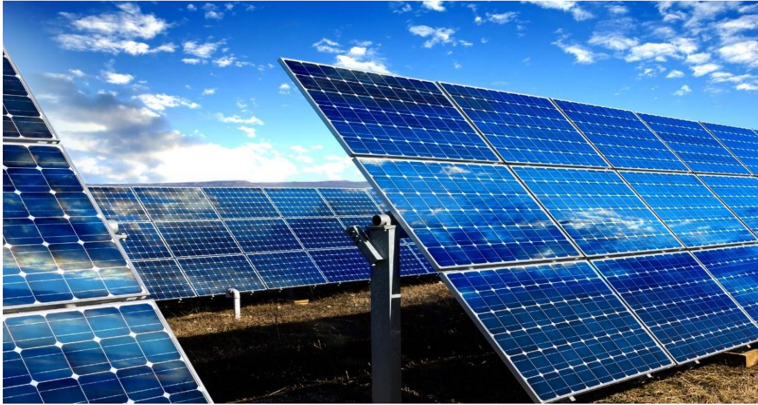
Figure 2.1. Solar panel field.
