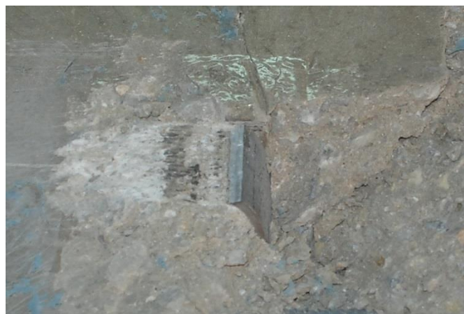
Figure 1.17 Channel Fracture – Concrete Slab
