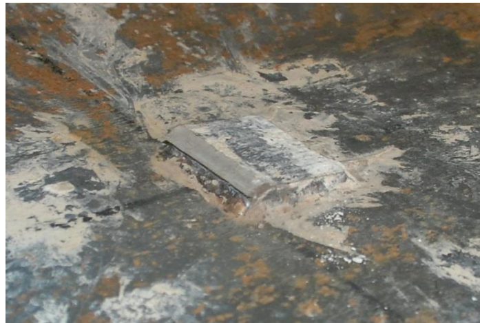
Figure 1.16 Chanel Fracture – Base Plate
