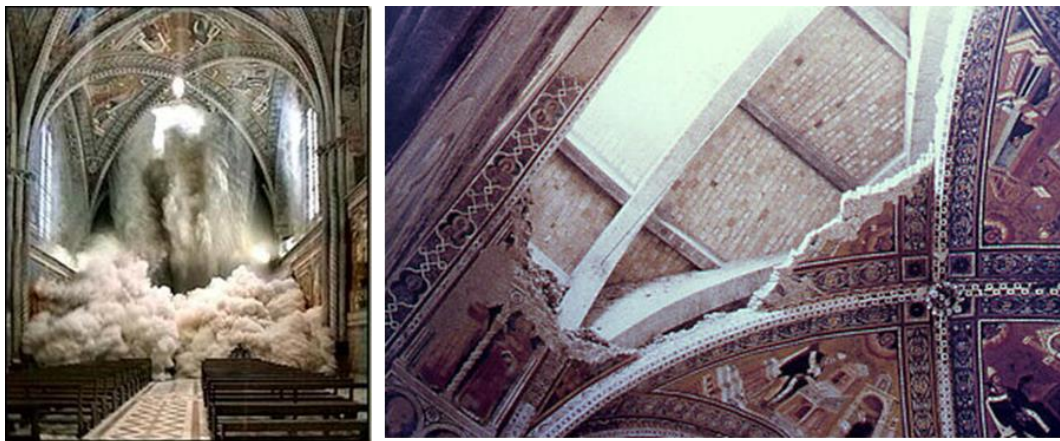
Figure 3.2. (a) The instant that the collapse occurred during the second event (left), (b) the collapsed vault (right)
