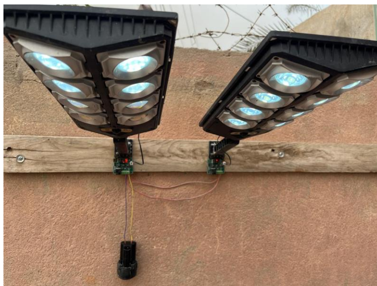
Figure 5.4. Image of solar panels working in wintter season.
