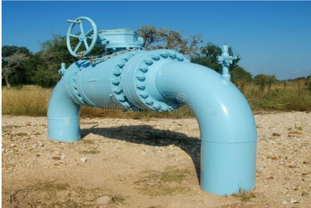
Figure 2.17 : Pipeline Control Valve
