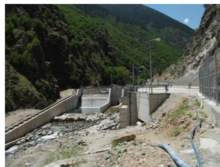
Borusan Yedigöl Plant
