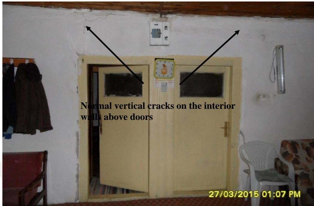
Figure 4.9 Normal vertical tension cracks above the door corners in the first floor of Sami Yıldırım's house (Bilgin et al., 2015)
