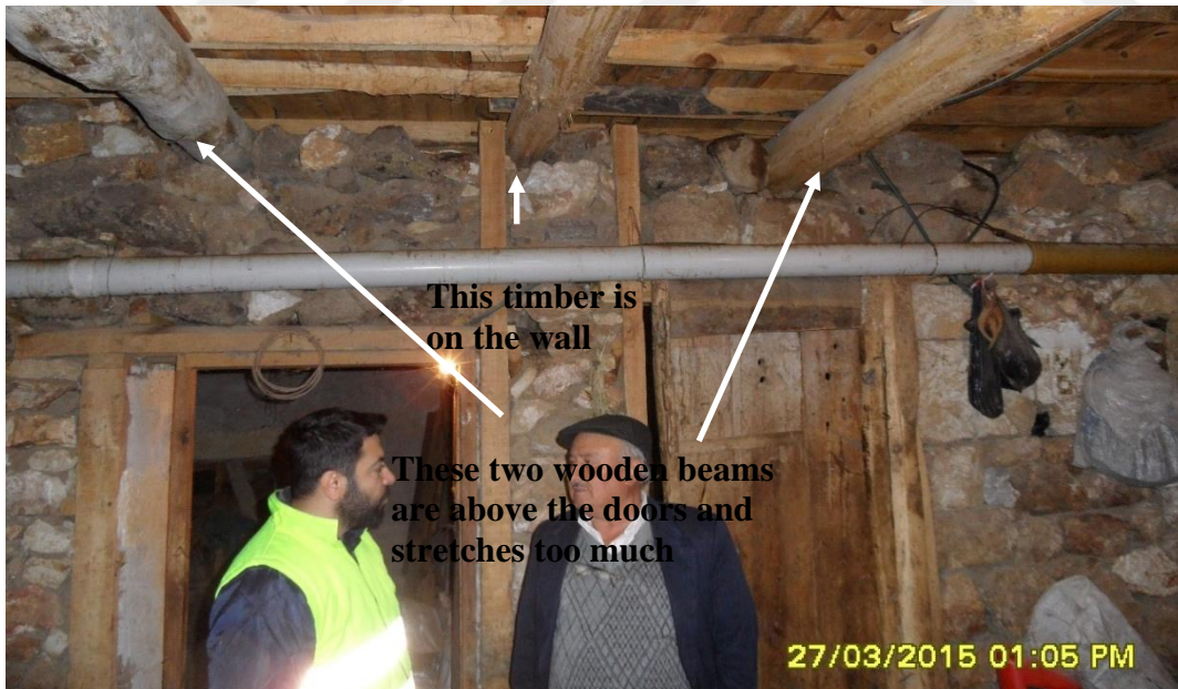
Figure 4.8 Mud-mortared walls and wooden beams in the basement of Sami Yıldırım's house (Bilgin et al., 2015)
