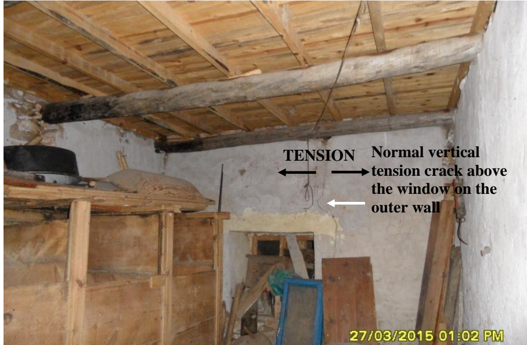
Figure 4.10 Normal vertical tension crack above the window in the basement of Sami Yıldırım's house (Bilgin et al., 2015)
