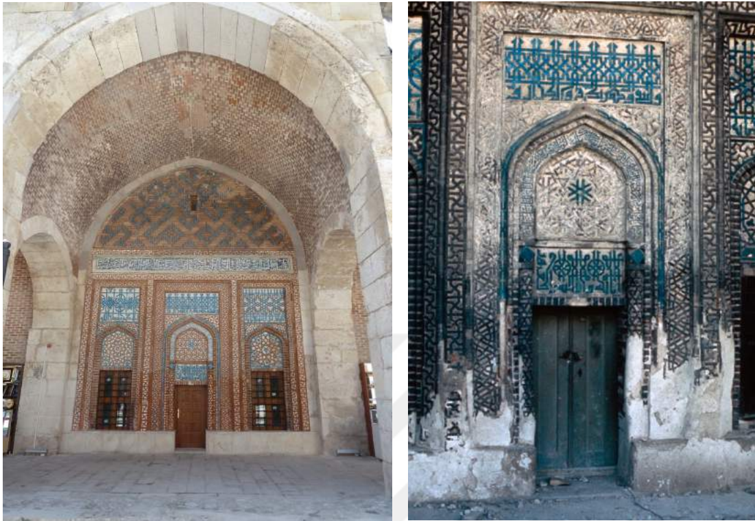
Figure 3.4 : Left: Entrance portal of the Keykavus Tomb, in Şifaiye Madrasa, 1217-1218 A.D. (Photo Credits Right: Aslihan Erkmen). Right: Close-up before the recent restoration (ca. 1960) (Photo taken from the “Aga Khan Visual Library” (n.d.)). The structural element is a combination of cut-stone and brick.
