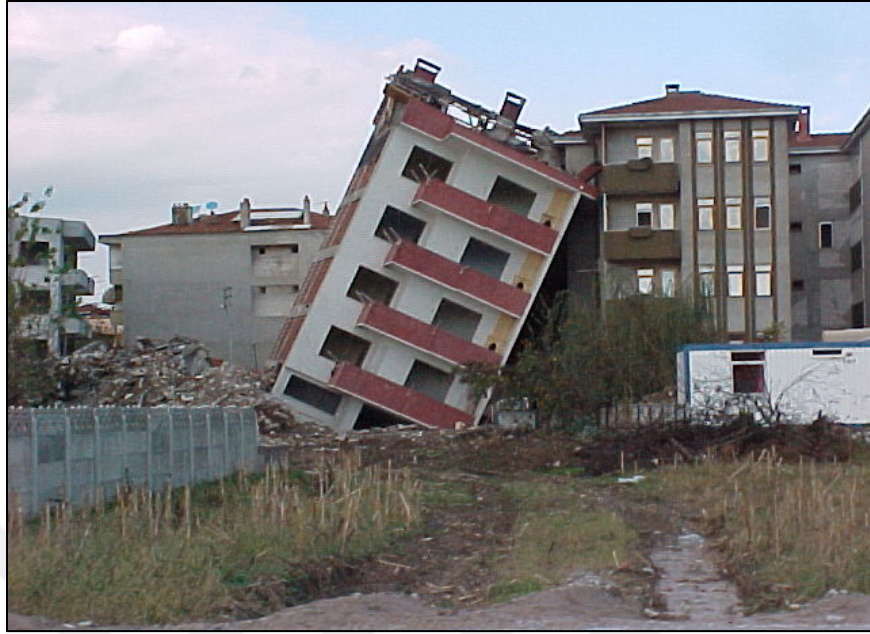
Figure 2.5 Liquefaction-induced bearing capacity failure due to lack of shear strength, The City of Adapazari [46]
