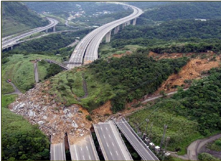
Figure 2.6 Taiwan landslide slope failure [47]
