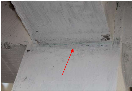
(a) First flexural crack in the columns
