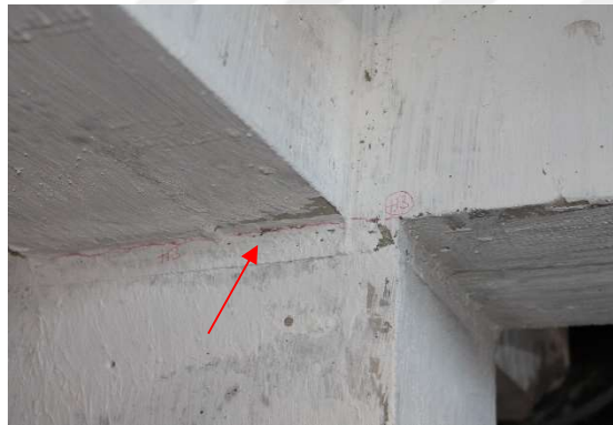
(a) First flexural crack in the column
