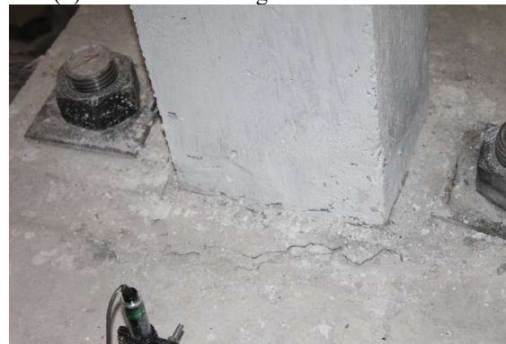
(d) Swelling of concrete at +2% drift ratio
