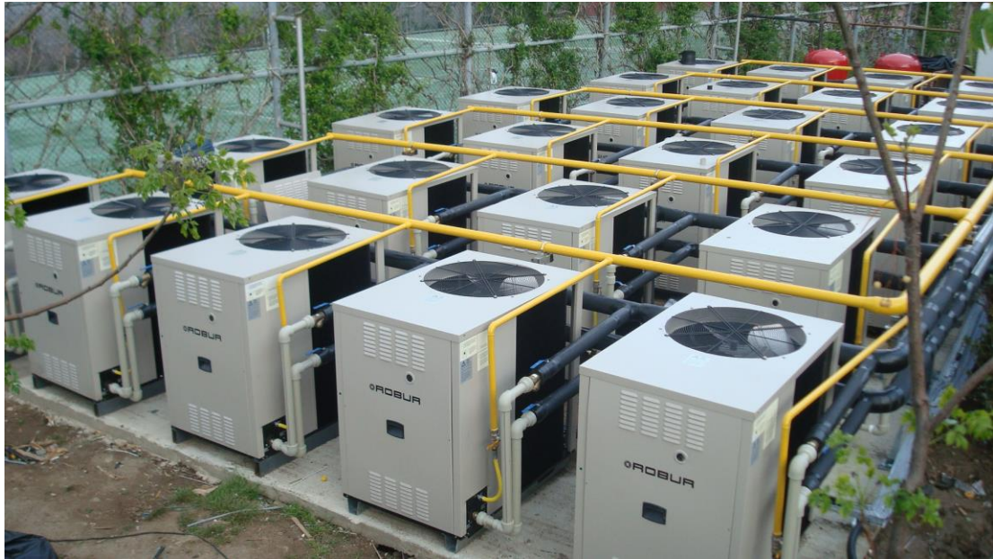
Figure 2.6 GAHP units outside installation view
