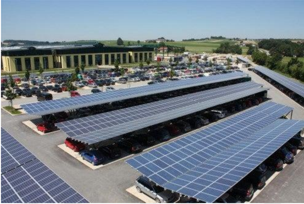
Figure 10. An example of a solar parking lot arrangement [21].
