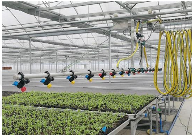
Figure 3.6. Irrigation System and Filter Systems for Sample Greenhouse Design (Courtesy of Emre İçöz)
