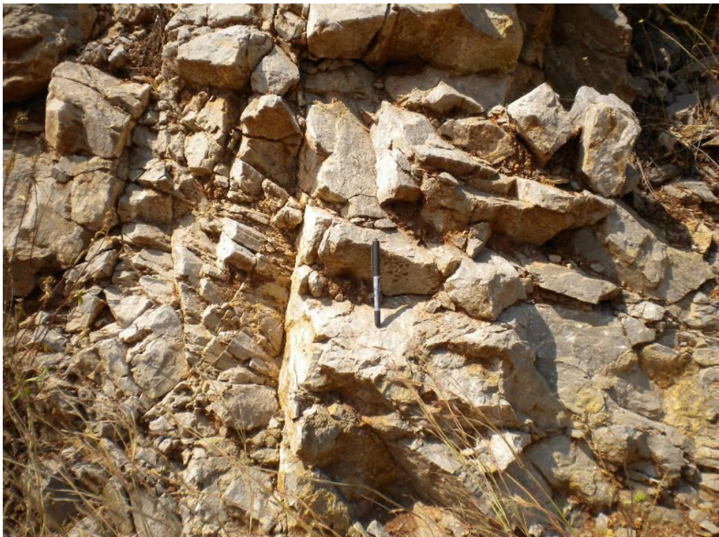
Figure 3.21. Discontinuities developed in the limestone at Km: 26+000.
