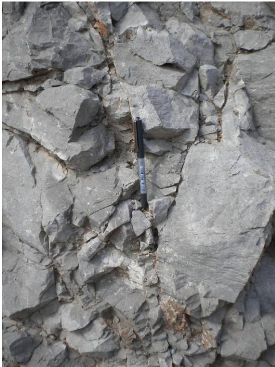
Figure 4.11. Photograph showing main discontinuities developed in the limestone at Km: 26+000.
