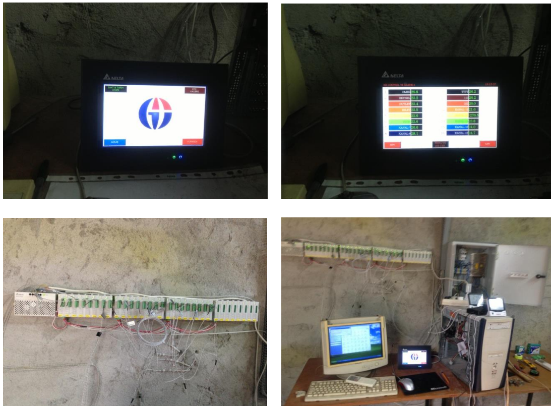
Figure 4.6. Data loggers and connector modules with PC for data measurement
