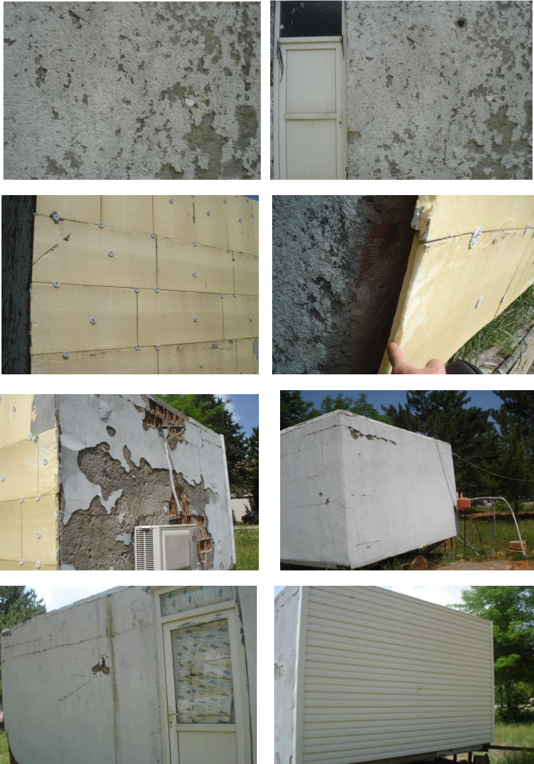
Figure 4.3. Case of walls of two testing room before maintenances
