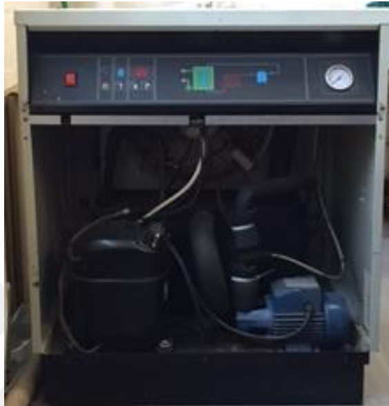
Figure 3.6 Photograph of the chiller unit.
