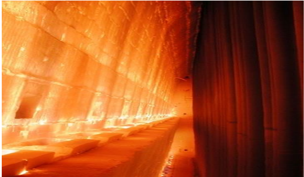
Figure 2.3. Inside of Terrace Wall TM steam reformer radiant box.
