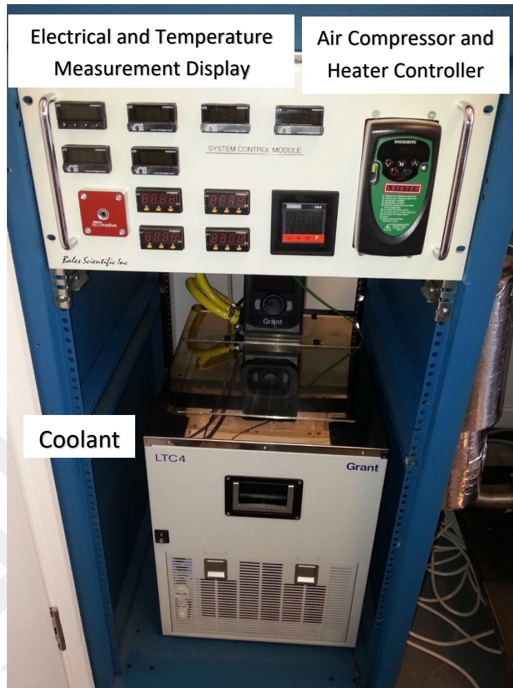
Figure 7-18 Coolant and first data acquisition unit.
