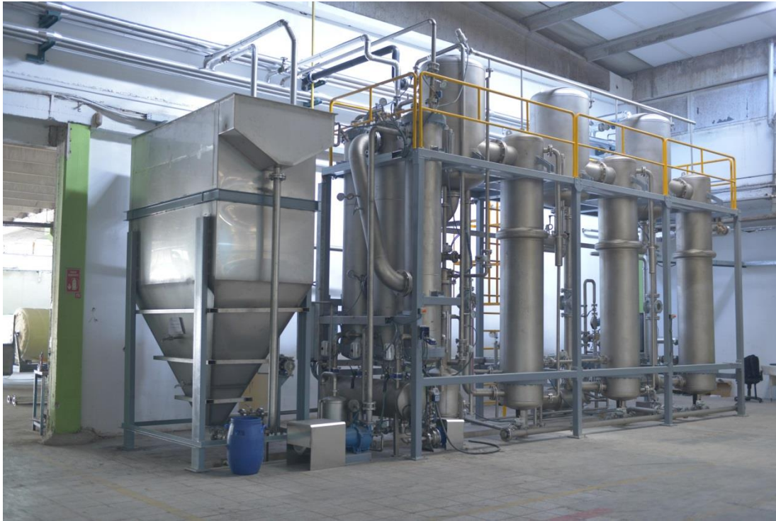
Figure 10. Evaporator in the Study Plant 2 in Denizli
