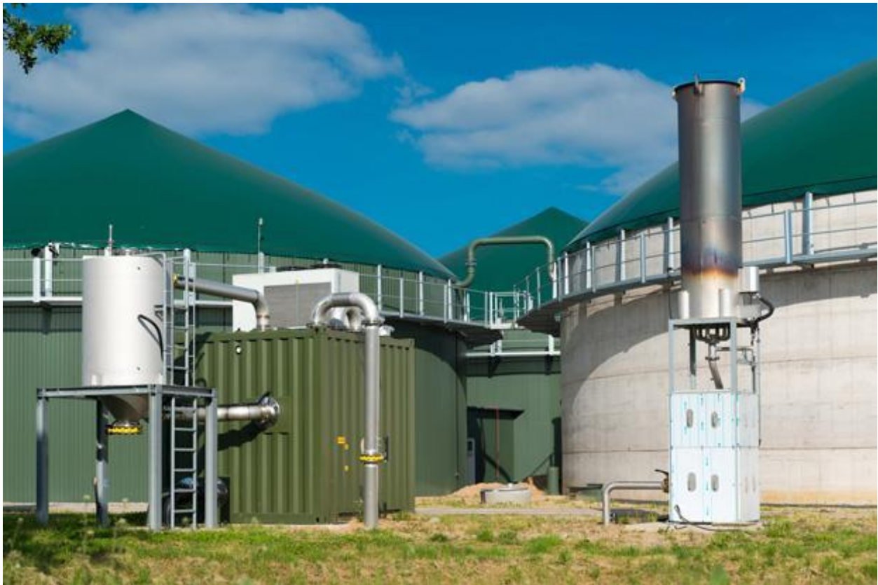
Figure 3.4 : Samsun Avdan Energy Landfill Power Plant.
