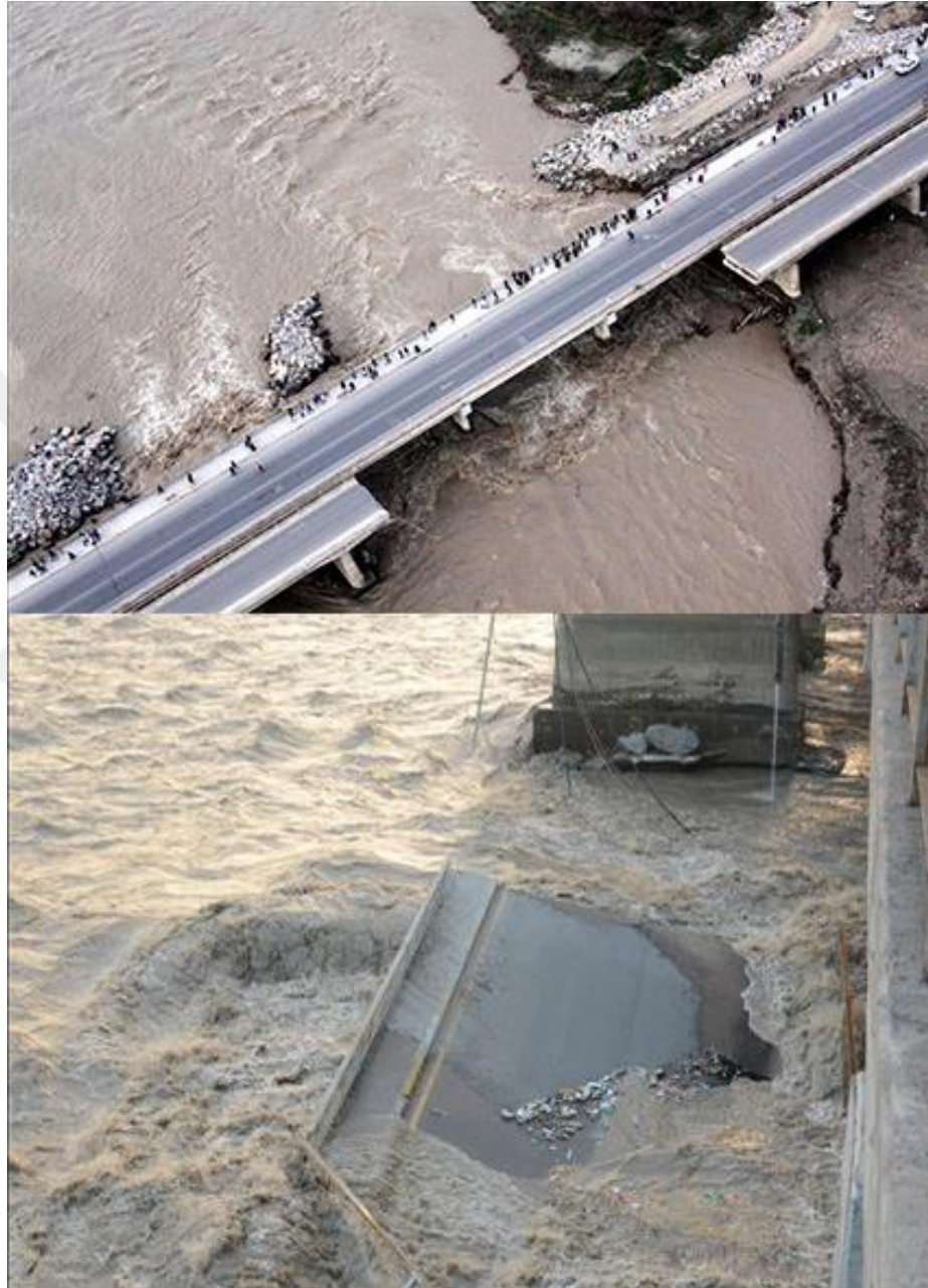
Figure 1.1 The failure of the Çaycuma bridge in Zonguldak Province, which is located near the Black Sea in Turkey (April 2012). The source of the pictures is the Anadolu Agency (Ajansı).
