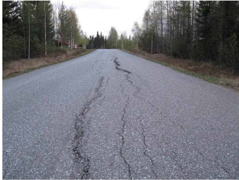
Figure 2.4 : Asphalt road damage due to swelling soils.
