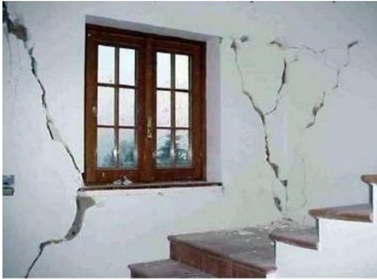
Figure 2.2 : Cracks on wall of a building due to upward soil pressures.
