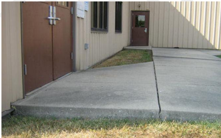
Figure 2.1 : Heave of concrete slabs adjacent to industrial building.
