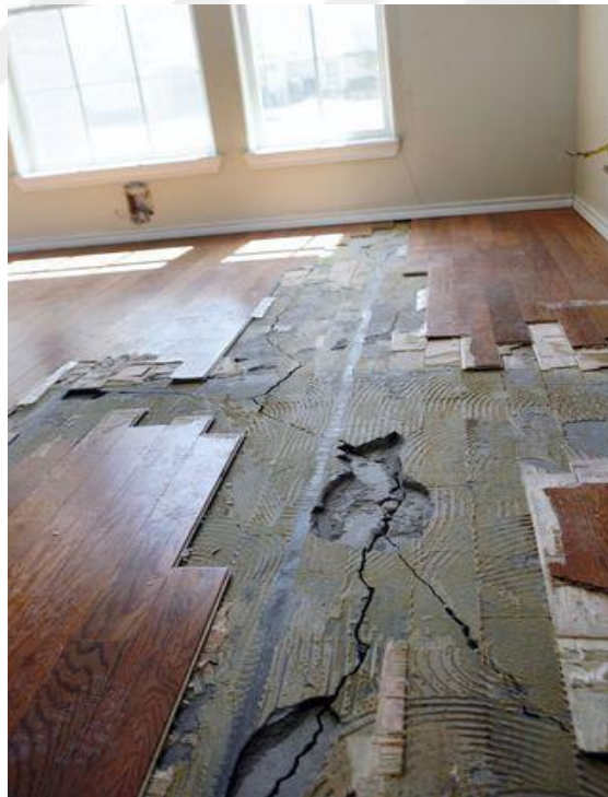
Figure 2.3 : Damage at a ground floor due to expansive soil.
