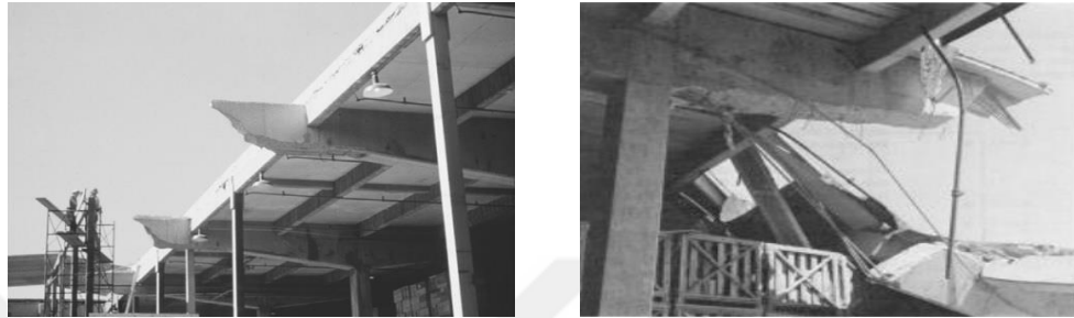
Figure 3.1 Shear failure of 914 mm deep beams in Wilkins Air force warehouse (Ohio,1955)
