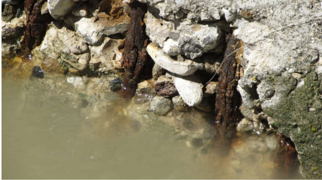
Figure 2.16: Example of Corroded Reinforcement (Özdemir and Topkara, 2015)
