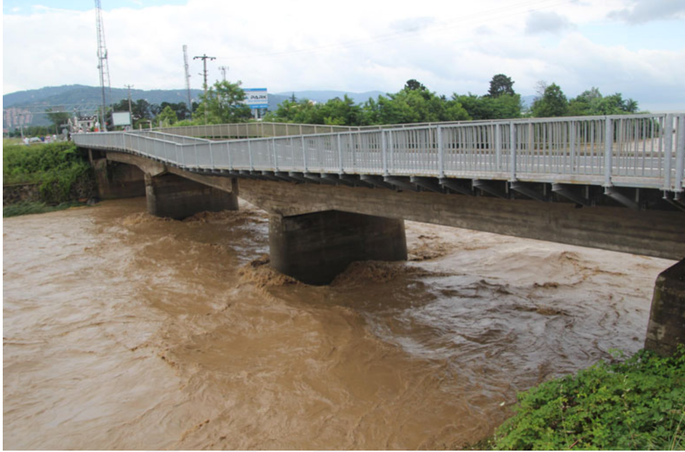
Figure 1.2. Damaged view of Akçaova Bridge in July, 2016 (Sozcu, 2016)
