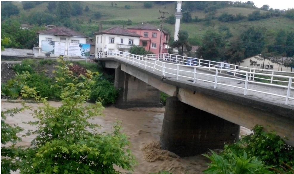
Figure 1.3. Damaged view of Karşıyaka Bridge in May, 2016 (İleri, 2016)
