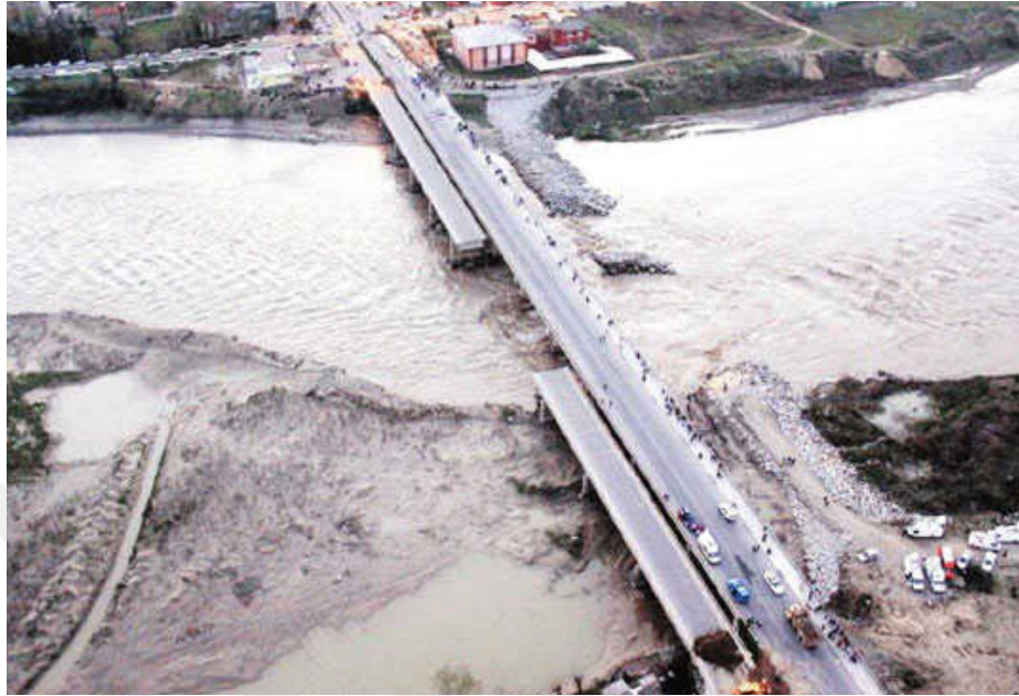
Figure 1.4. Collapsed view of Çaycuma Bridge after flood in 2012 (Sondevir, 2012)
