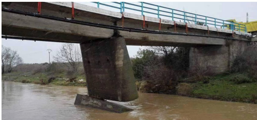
Figure 1.1. Yayakent Bridge view after flood in January, 2016 (Tuna, 2016)
