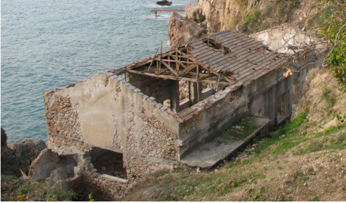
Figure 35 Energy Power Plant (source: Antalya KUDEB)
