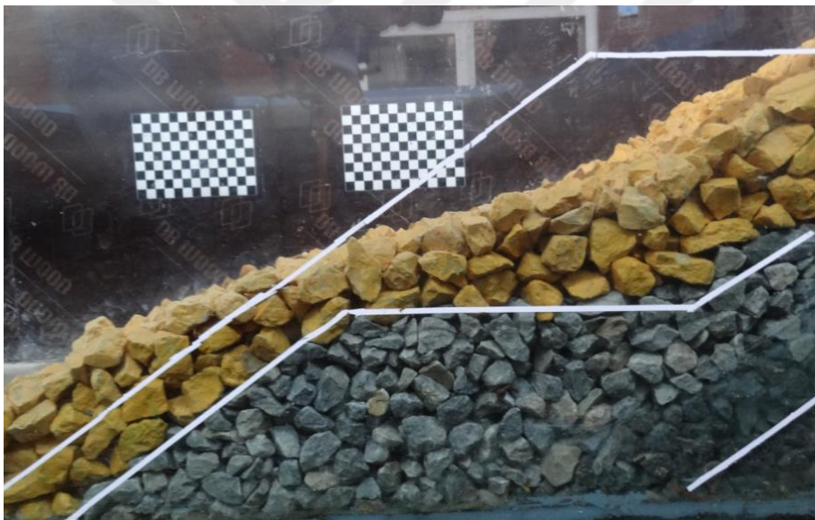
Figure 4.12 View of Section 2 after set 1 (1000 waves)
