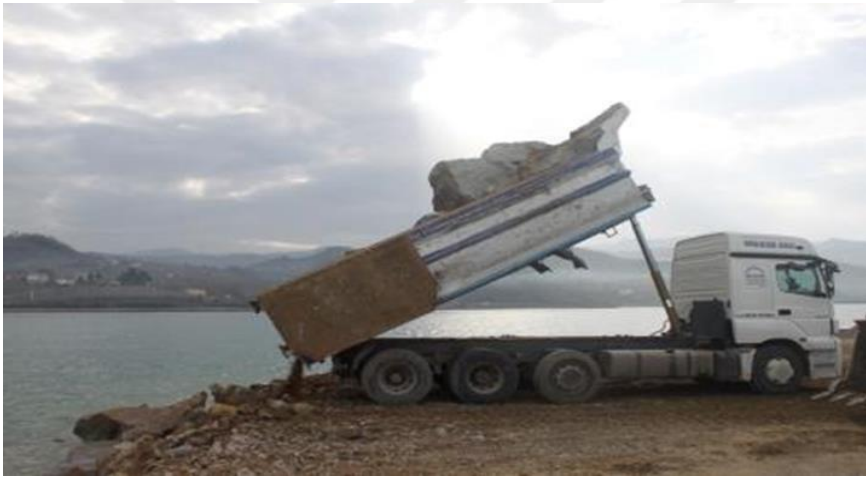
Figure 4.44 Unloading of stones into the sea, Retrieved from İbrahim Ahmetođlu, Project Manager of Cengiz Insaat.
