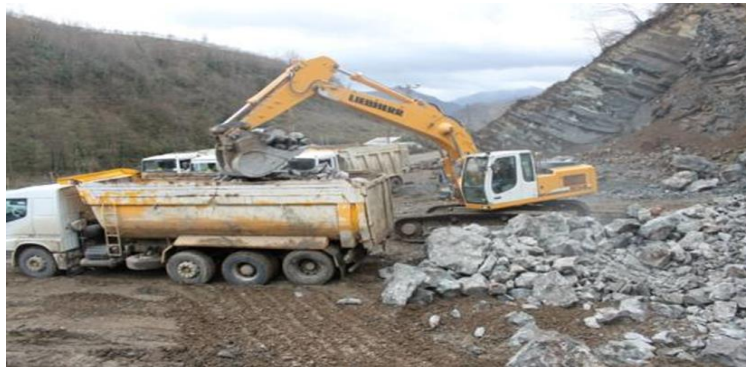
Figure 4.42 Loading of stones, Retrieved from İbrahim Ahmetoğlu, Project Manager of Cengiz Insaat.
