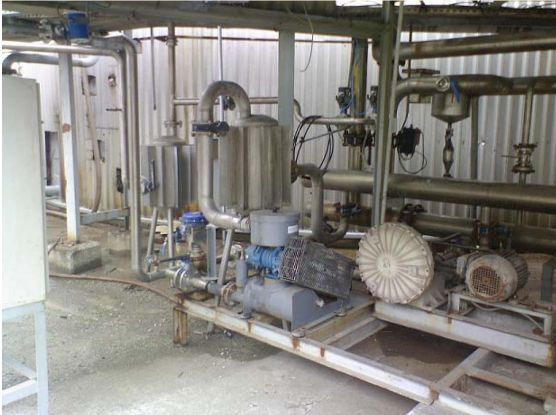
Figure 3.3: Biogas compressor and Moisture trappers
